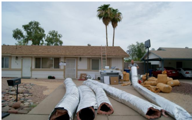
Flex duct for new HVAC air delivery system waiting for installation
