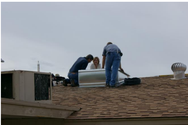
Chairman Mayes looks on as contractor Al Lopez talks about the benefits of new HVAC system.
